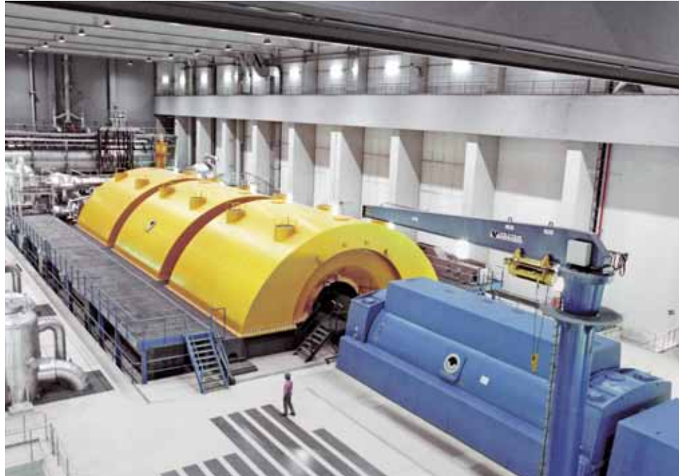
SST5-9000 steam turbine in the nuclear power plant (NPP) in Unterweser, Germany
